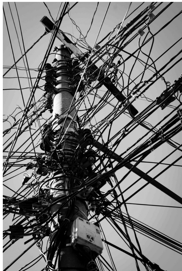
Fig. 1. Illegal electricity extensions on a pole, also called gambiarra . (Photo © J.P. Oliveira)
